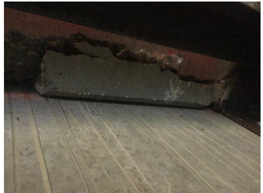
Damage to panel 1 at right approach
