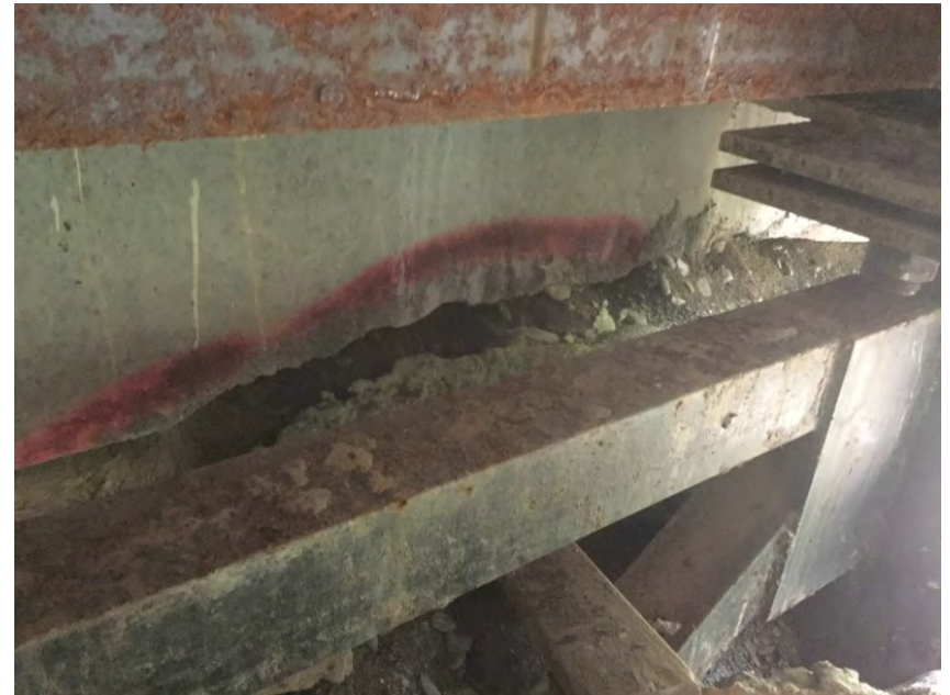
Damage to ballast wall at left approach
