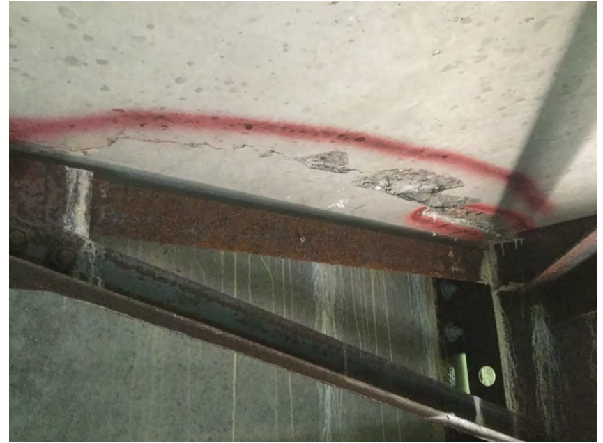
Damage to panel 1 at left approach
