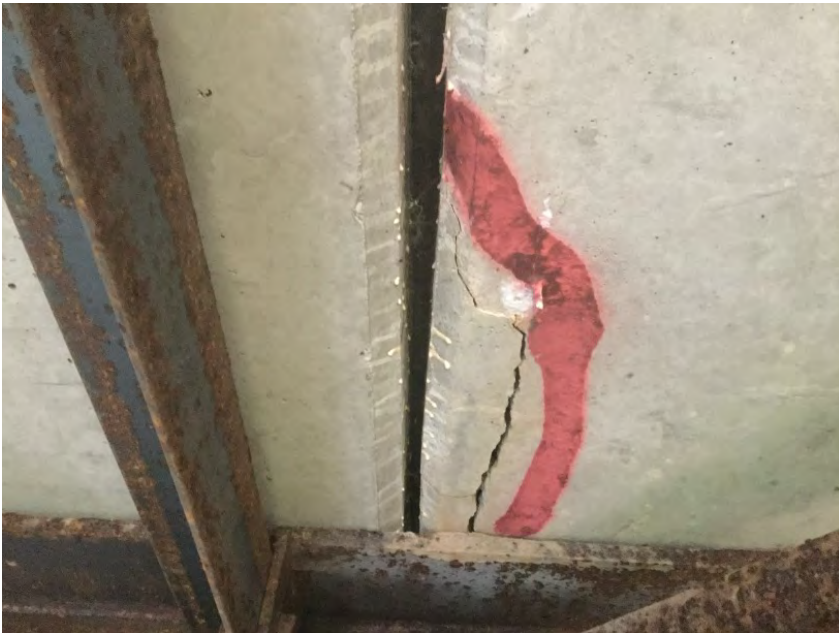
Damage to panel 1 at left approach
