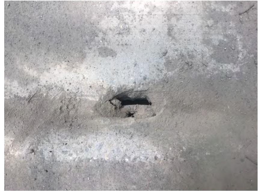
Damage to ballast wall and deck panel at left approach
